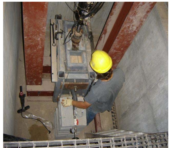
David in 2007 performing hydrofracture experiments using the small buried pipe test cell.
